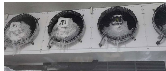
General air cooler
