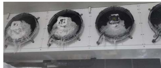
General air cooler
