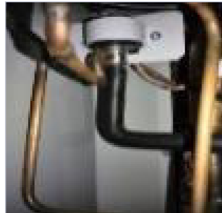
Low temperature spray design to improve operation reliability
